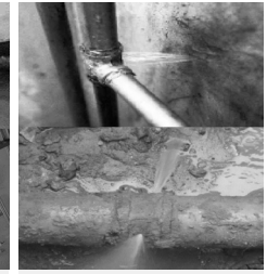
Fire Sprinkler System
