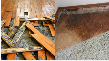
Leak Under The Floor
