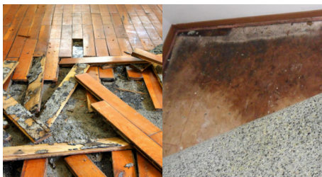
Leak Under The Floor
