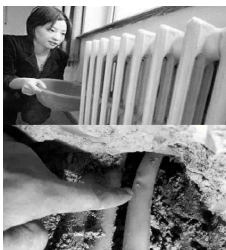
Heating Pipes/ Underfloor Heating Pipe Leaks
