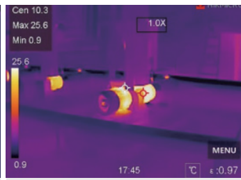
Check Machine Temperature
