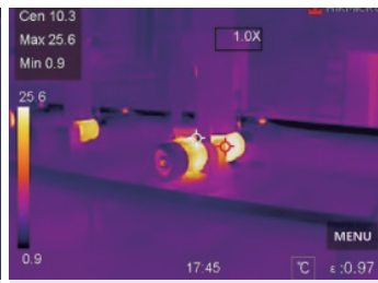
Check Machine Temperature
